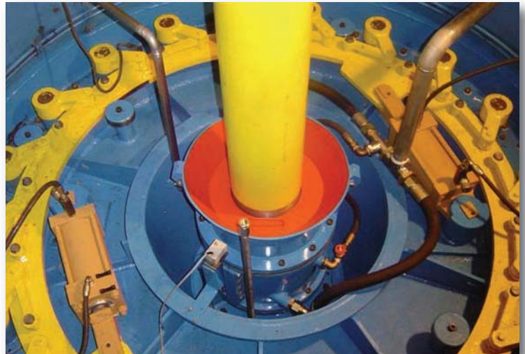
Thordon SXL main guide bearing installed at Graus Power Station, Spain
